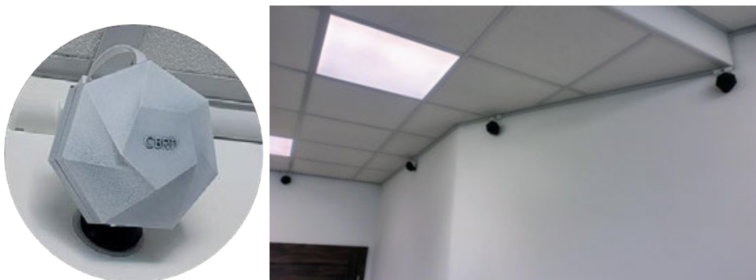
Fig. 1. A close-up view of the reflection probe (left) and an overview of the ceiling-mounted structure of the entire reflection tomography system (right)
